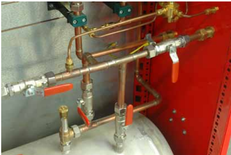
Fig.: Bypass for buffer vessel, blow-off pipe
