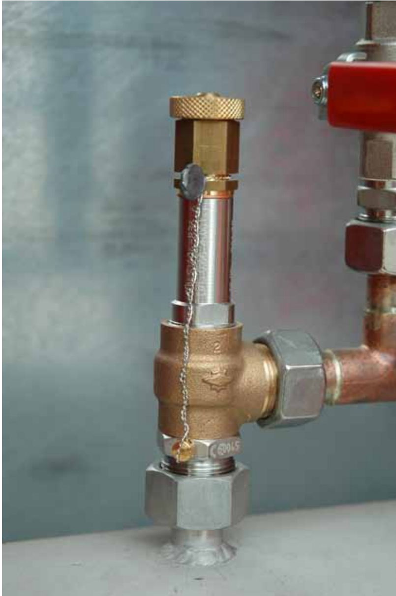
Fig.: Safety valve for buffer vessel
